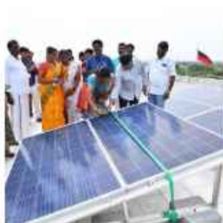
SOLAR ELECTRIFICATION STATION
